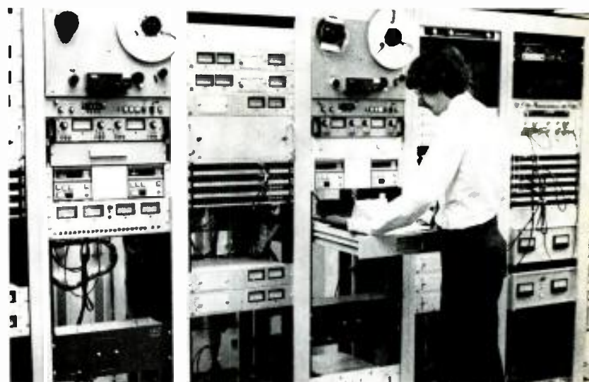
Chief engineer David Pollard makes adjustment in terminal room of new RKO network plant. Racks hold audio processing and amplifying equipment, cart and reel players, patch panels. Room can go on air if needed
